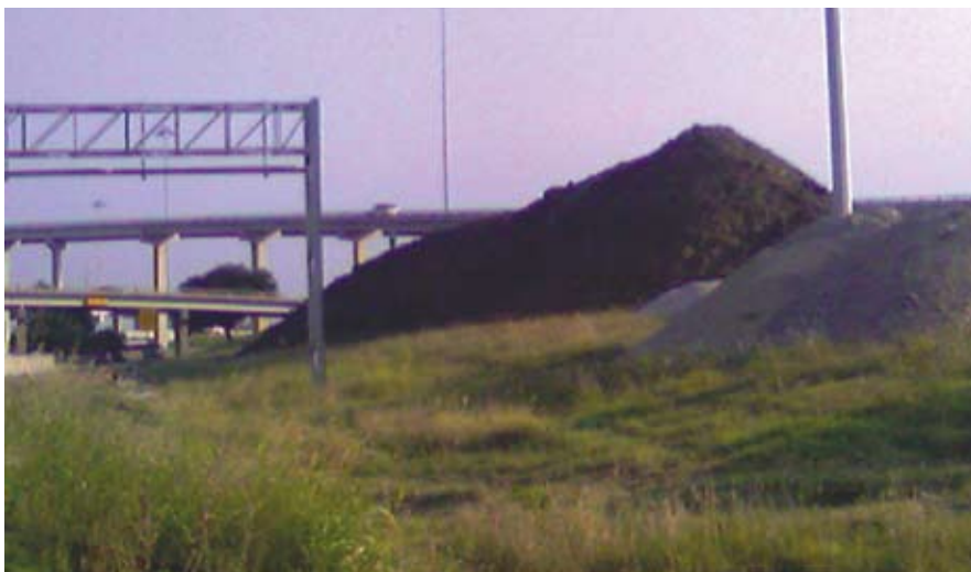
It required 1,500 soil samples to determine what soils could be recycled. The XRF equipment efficiently allowed the contaminated soil to be identified and stockpiled for proper disposal.
