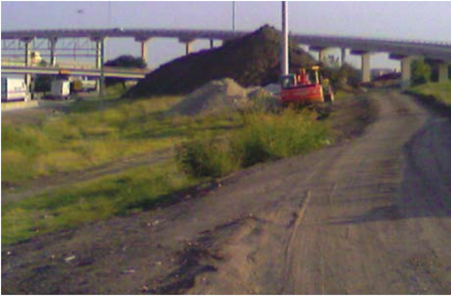
Soil tests at the construction site found that some of the soil was contaminated with metals and could not be used. Excavated soils had to be stockpiled until a determination allowed the soil to be properly disposed or reused on the project.
